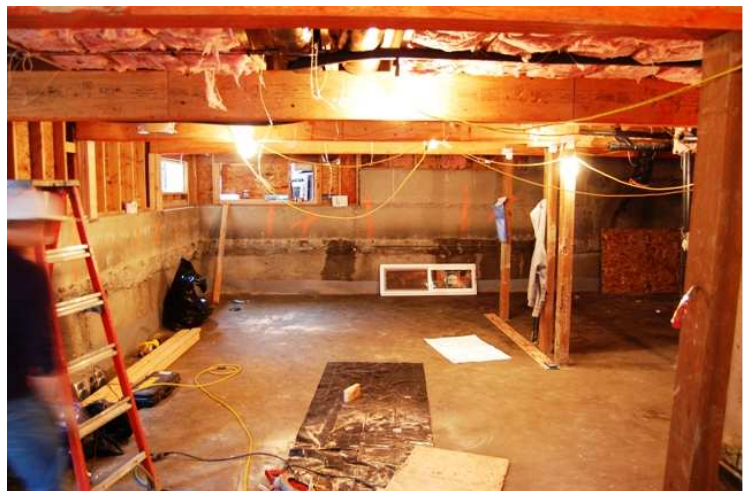
6- Install concrete in the open segments and remove soil to final basement grade.
