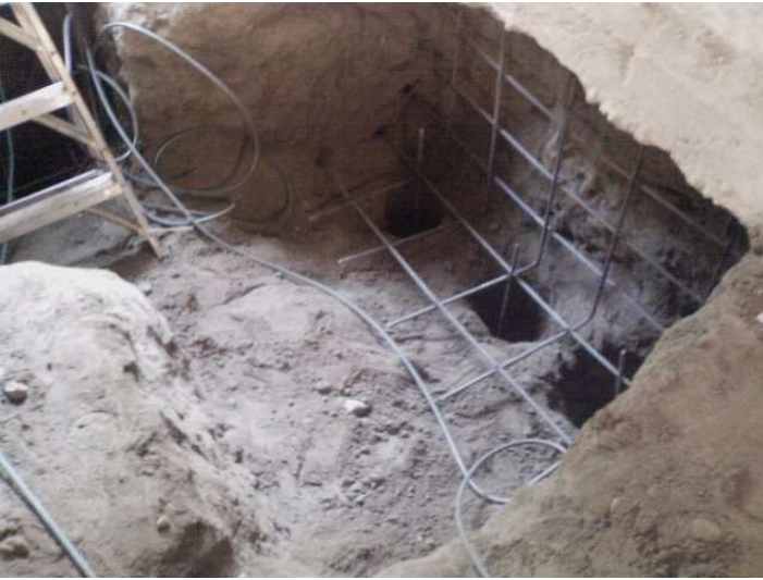
3- Install piles and rebars and extend horizontal rebars to future 5 ft segment wall in soil.
