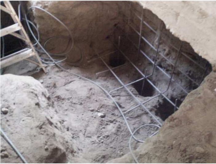
3- Install piles and rebars and extend horizontal rebars to future 5 ft segment wall in soil.
